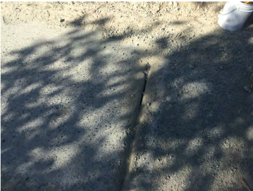
Failed Deck Panel Sealant at Left Abutment
