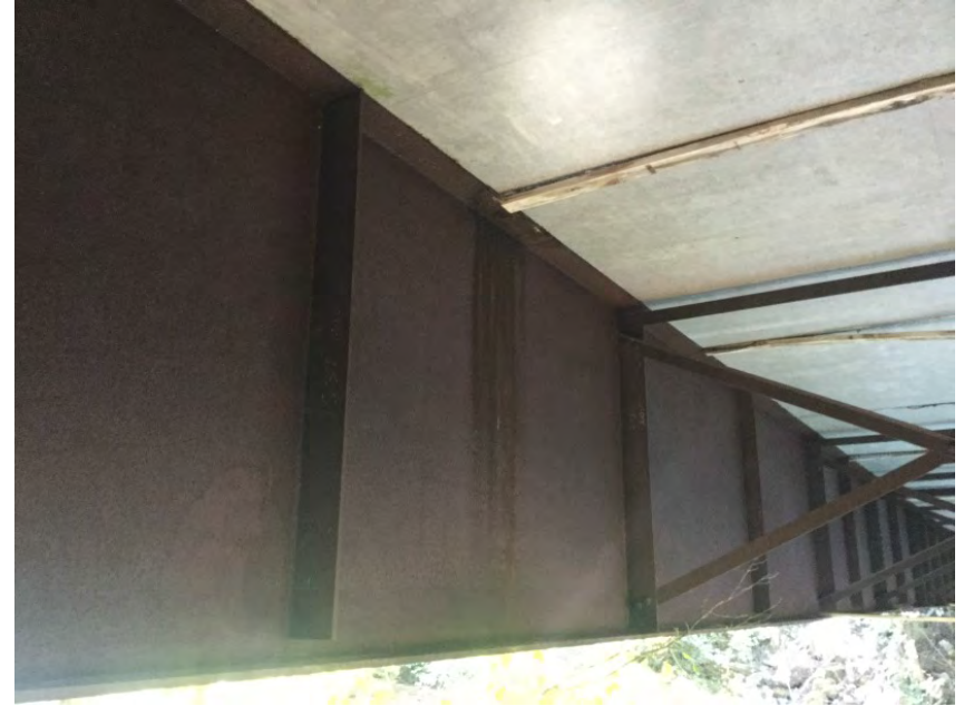
Corrosion of Girder at Panel Joint
