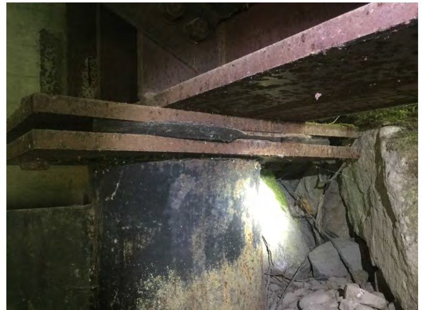
Typical Bulging Bearings
